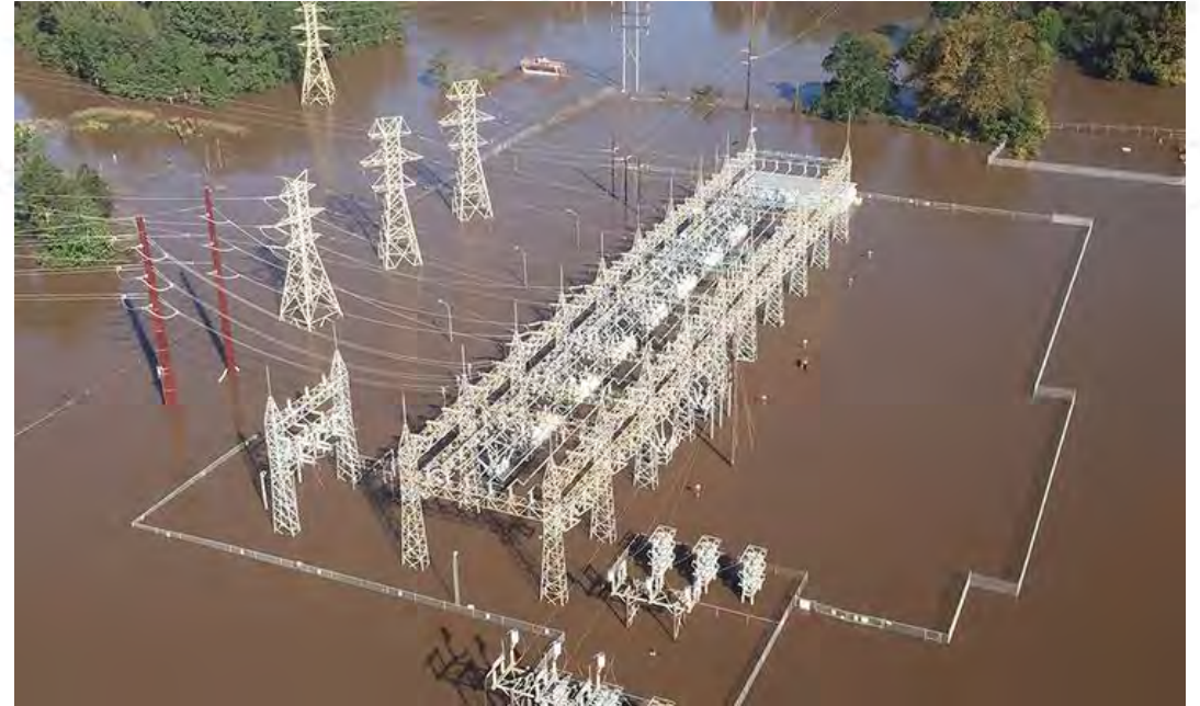
Substation in NC after Hurricane Florence
