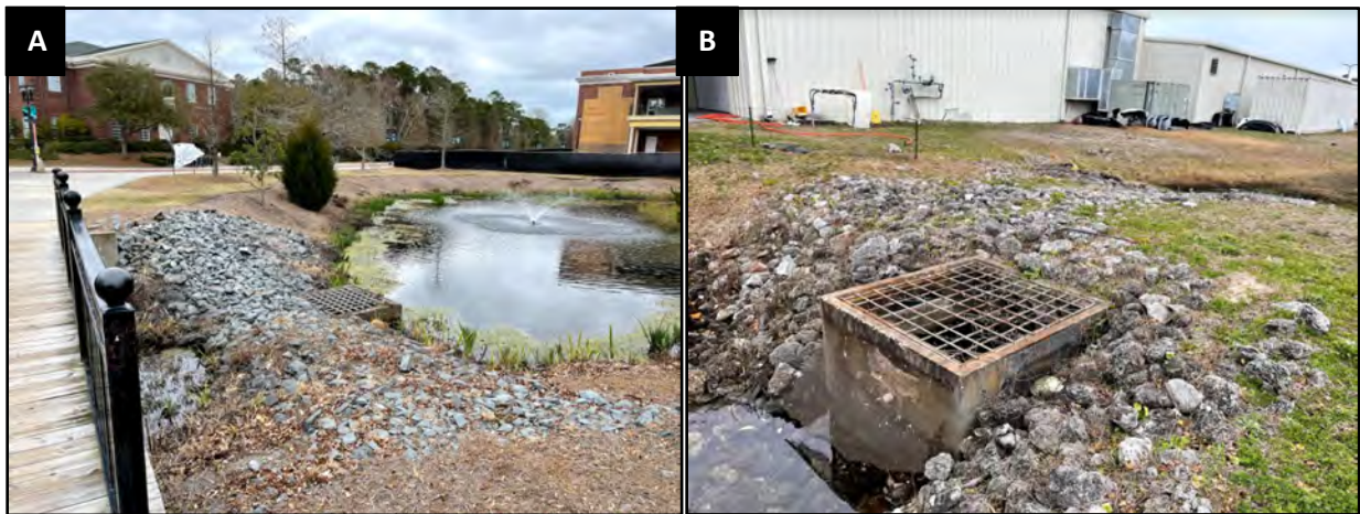
Figure 3. Design Fundamental: Accessible outlet structure on well armored berm. A. Well armored access berm for outlet structure. B. Well armored access berm for outlet structure.
