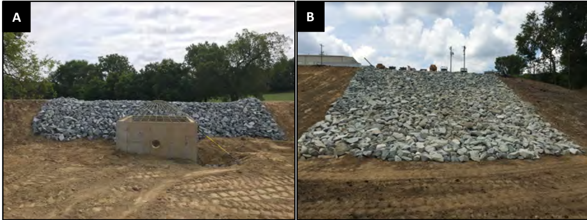
Figure 5. Design Fundamental: Overflow (emergency) spillway well armored and below top of berm. A. Spillway is sufficiently below the top of berm and rip rap extends below the normal pool. B. Spillway armament extends to toe of berm slope.
