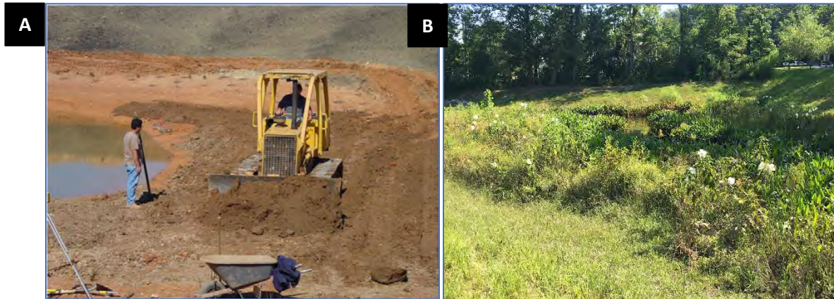
Figure 6. Construction Fundamental: Establishing stable vegetation cover is key to resiliency. A. placing a plant-friendly soil over a compacted berm helps create B. conditions supporting a thriving vegetative community.
