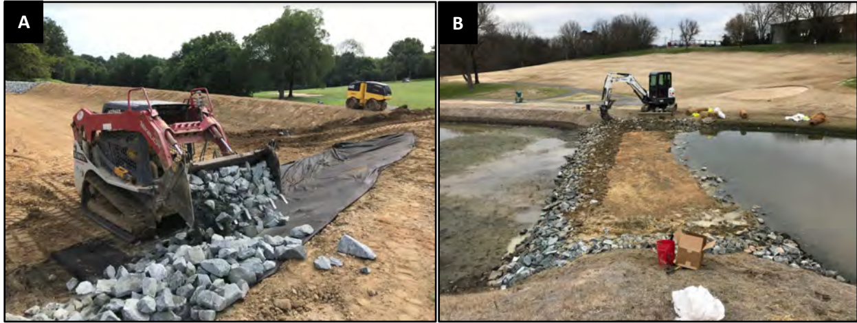
Figure 2. Design Fundamental: Well-armored forebay berm. A. Well-armored primary flow path – side slope of berm – with nonwoven geotextile. B. Coir geotextile keyed-in under rip rap and soil along secondary flow path – top of berm. Well armored internal flow path – upper berm.
