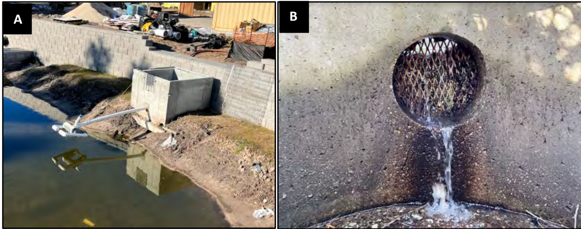
Figure 4. Design Fundamental: Redundancy of flow paths for trash racks and outlet structures. A. Four flow paths are present: a draw down skimmer orifice, an intermediate flow weir, an overflow weir, and an emergency spillway. B. Clogged low and intermediate flow orifice lacking redundancy and offset trash rack.
